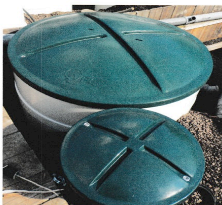
Figure 1: The system AT8 +P installed on the PIA testing field
